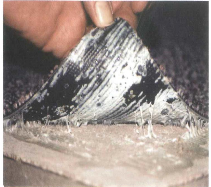
Figure 3-1. Due to excessive moisture and a high pH in the concrete surface, the adhesive under this vinyl backed carpet tile has reemulsified and has lost most of its holding strength. (IMG16042)
