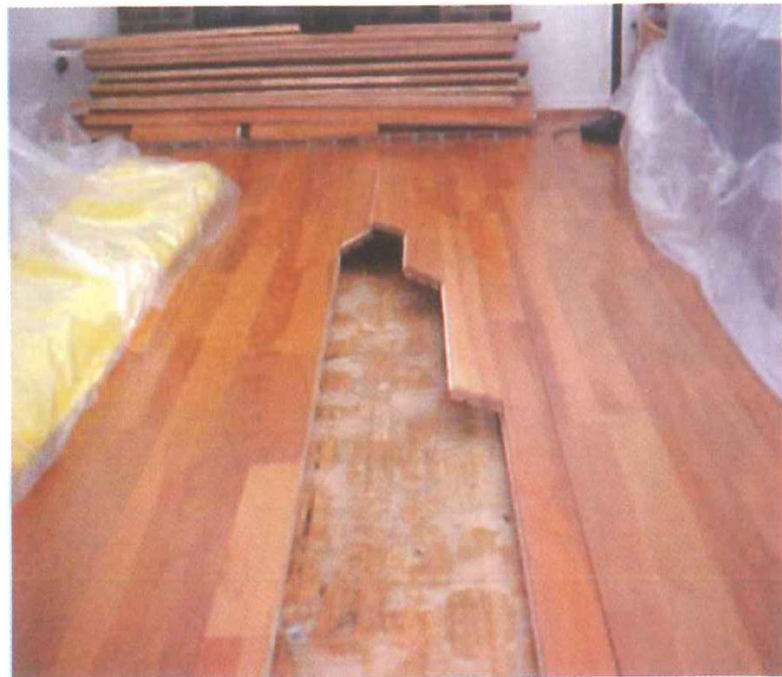
Figure 3-8. In this residence, wood flooring was glued directly to a damp concrete floor slab; the wood absorbed moisture from the slab, expanded, and buckled (photo courtesy of George Donnelly, Testing and Inspections).
