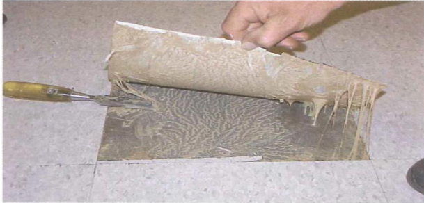
Figure 3-2. Adhesive oozing from joints (top) in recently-installed vinyl composition tile on a school floor. New tile (bottom) debonded due to moisture and high pH attack on new adhesive. (IMG16023, IMG16003)
