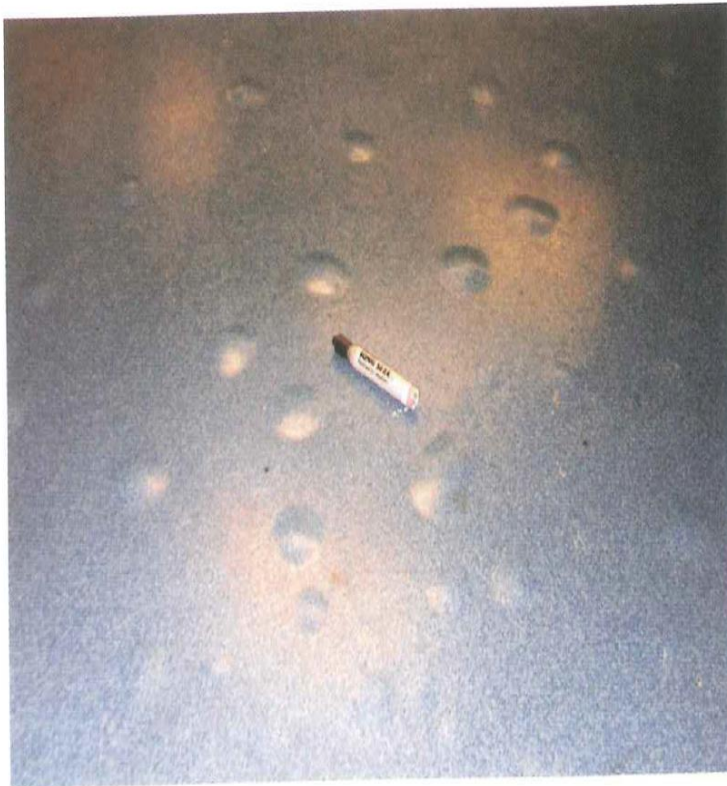
Figure 3-4. Osmotic blistering in epoxy floor coating (photo courtesy of Peter Craig, Concrete Constructives).
